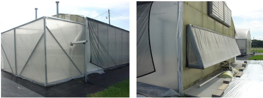
Fig 2. Insect screen covering air intake area.
